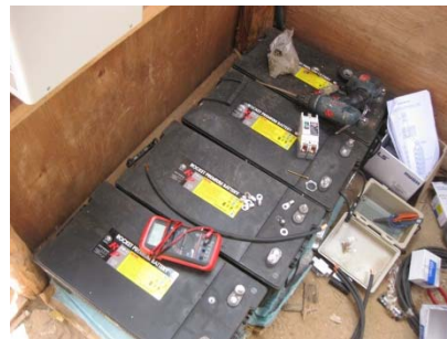
Battery 12[V] 1000[AH]
