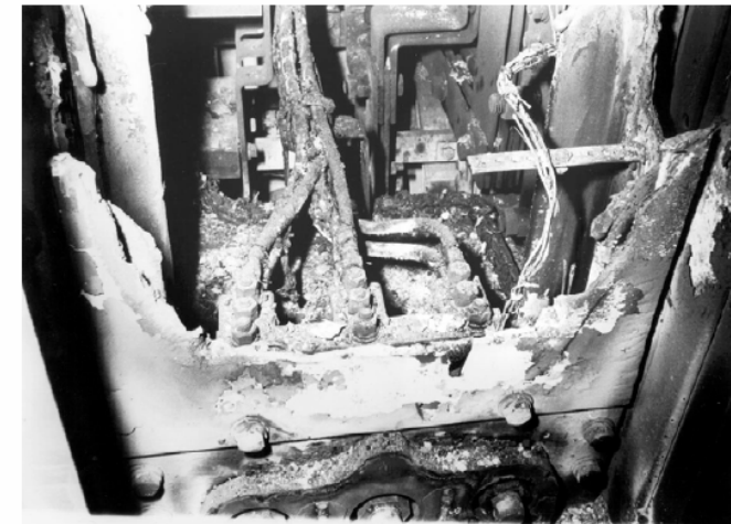
Figure 1. Arcing damage sustained on USS Parche (SSN 683). Note that some of the copper bus, cables, insulators, and switchboard structure are missing.
