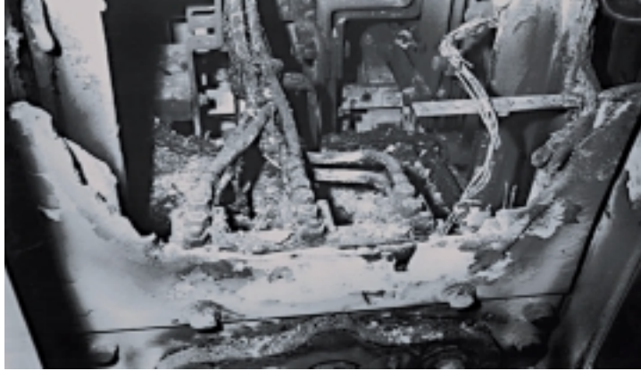
Figure 1: Damage from an arc-generated electrical fire (USS Parche (SSN 683)) 1
